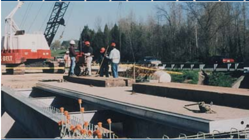
Little Buffalo Creek Bridge with its aluminum isotropic deck (on US Route 58 in Virginia) under construction in 1997
