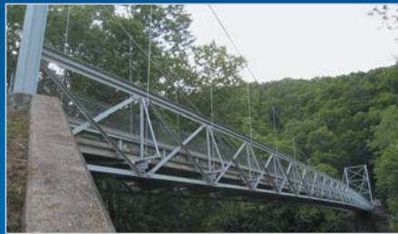
The historic Corbin Bridge in Huntingdon, PA with its nearly 13-year old aluminum orthotropic deck
