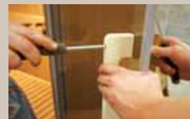
After about three hours work, it is time to screw on the door handle.
