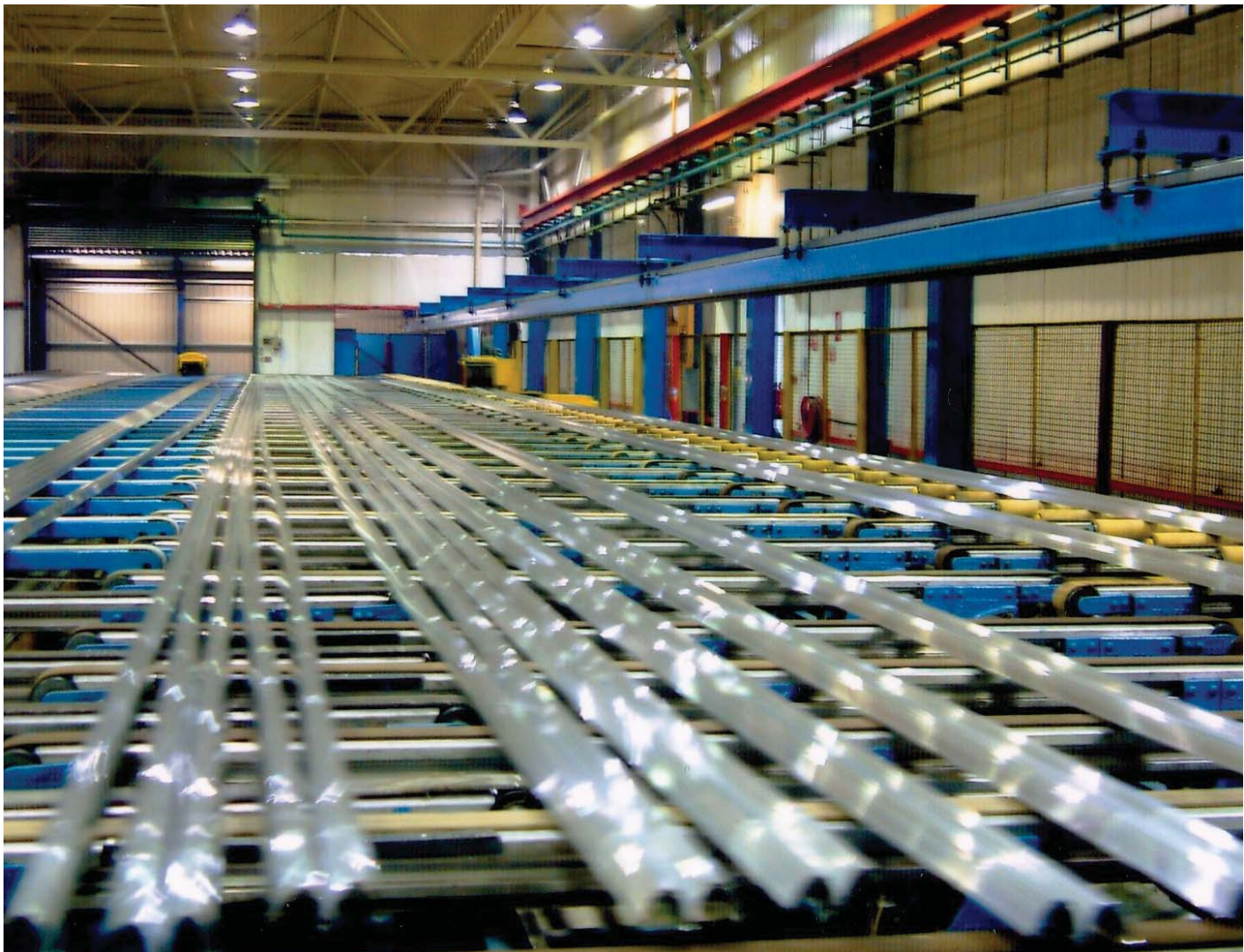
General view of the run-out table, part of the new press layout at Tibshelf
