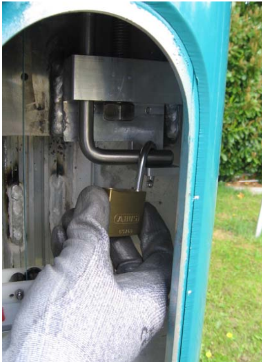
Pic. 19 Place the padlock, so it blocks the handle.
